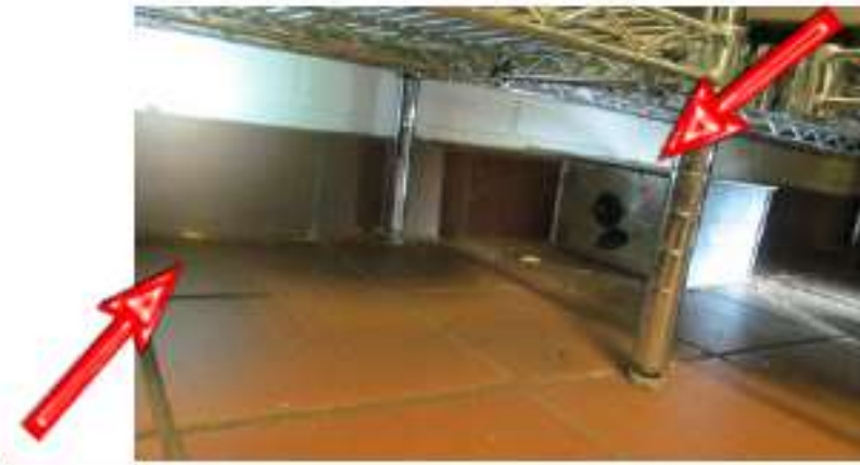
Image 1: Food debris and crumbs under food storage shelving. Also pictured on the right is the rodent trap where a mouse was found at the time of the assessment.
